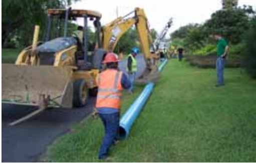
Figure 8: The backhoe's bucket center loads the previously installed length of pipe to keep it from moving while the new joint is being assembled
