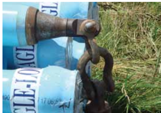
The contractor attached an 8-inch reamer directly to the pulling head and pipe.
