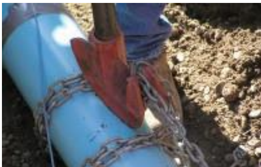
Figure 11: This assembly tool uses a chain wrapped around the bell and a lever bar to make the joint.
