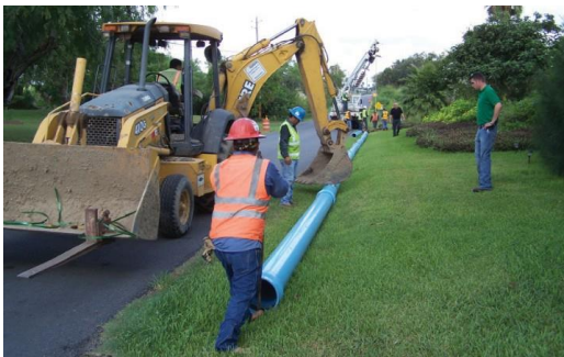
Figure 9: The backhoe's bucket center loads the previously installed length of pipe to keep it from moving while the new joint is being assembled
